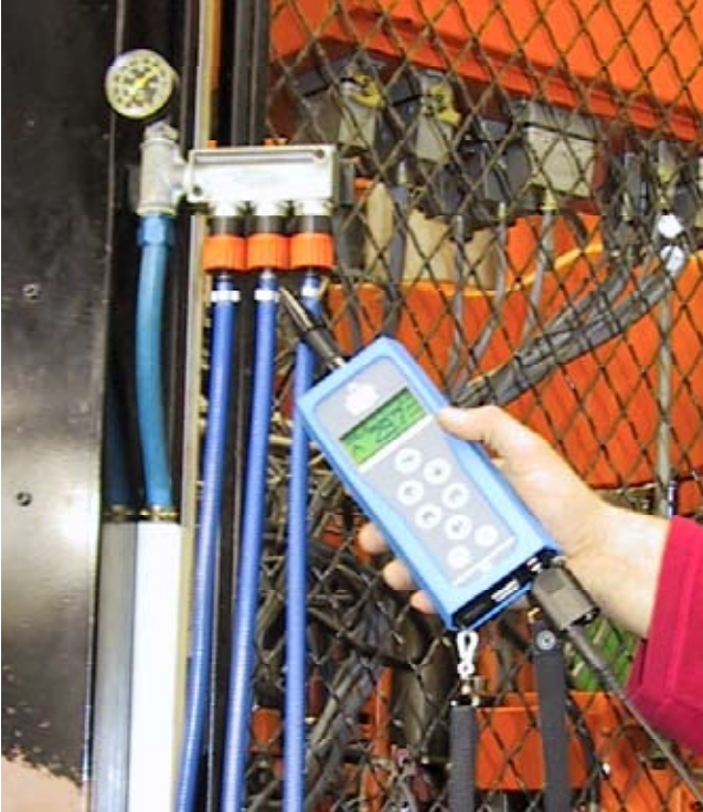
Image - The Internal Sensor is used here to find an easily accessible leak on a clamped air line.
