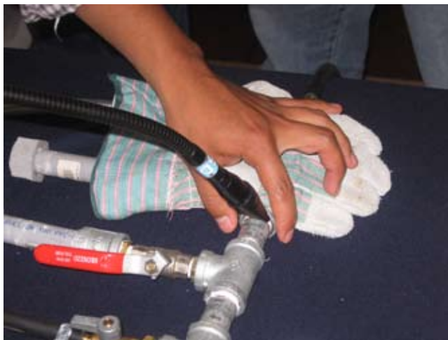
Pictured above, a simple glove is used to shield a leak
