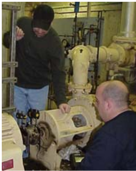
Mike Costa (left) and Bob Greatorex use laser alignment equipment on one of the pumps at the plant.
