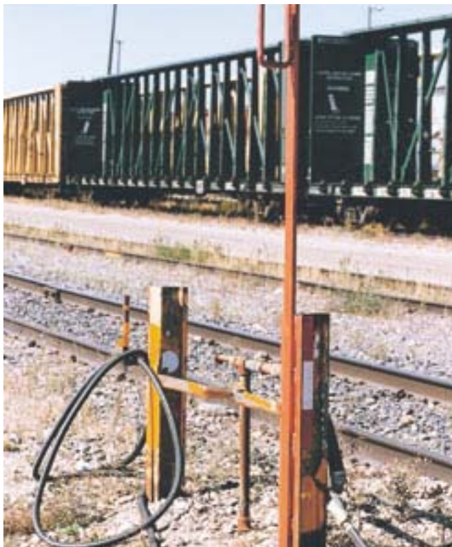
Compressed air "filling" station, for charging the braking systems on trains. Rails driven into the ground on either side of the risers protect piping from snow removal equipment.
