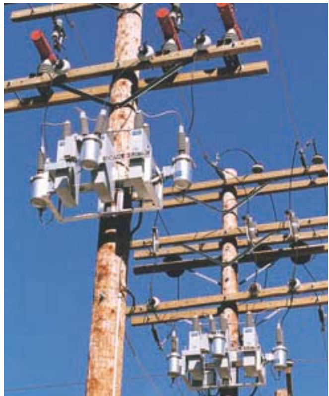
Power factor correction circuitry for entire load at the yard. The circuitry has two settings—one for winter and one for summer—for maximum year-round efficiency.
