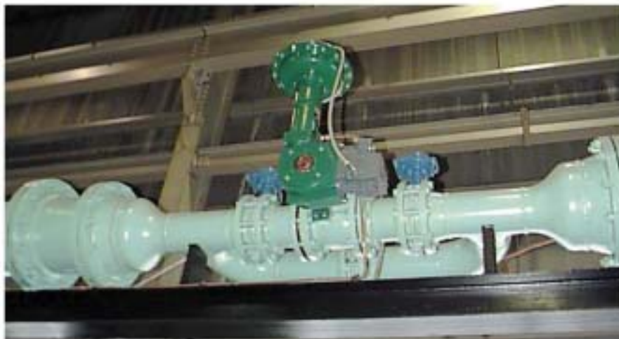
This control valve lowers pressure to reduce artificial demand.
