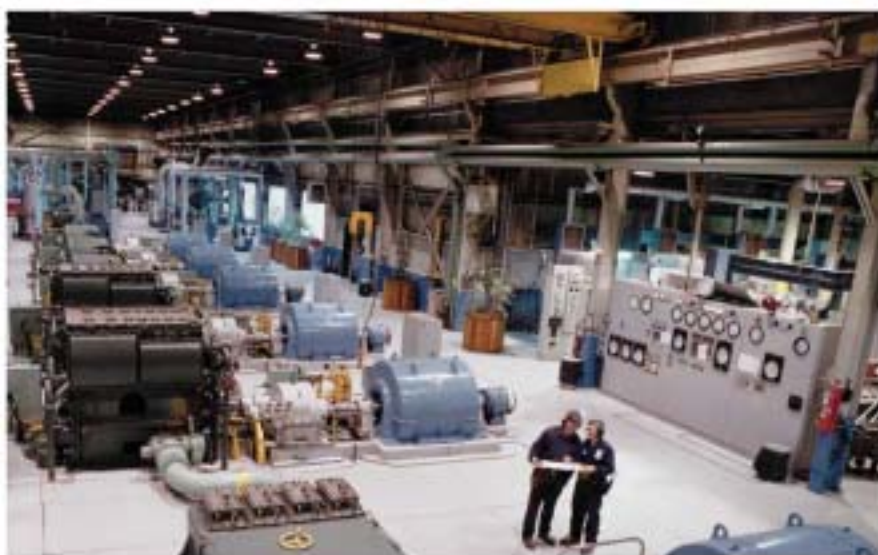
Powerhouse at Inco, with compressors totalling 23 000 hp. Compressed air from the powerhouse serves the mining complex through a network of pipes 13 km long.
