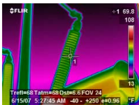
Figure 2 - Thermal images of A-phase bushing and incoming connection on this 161Kv to 13.8Kv step down transformer showed no apparent hot spots.
