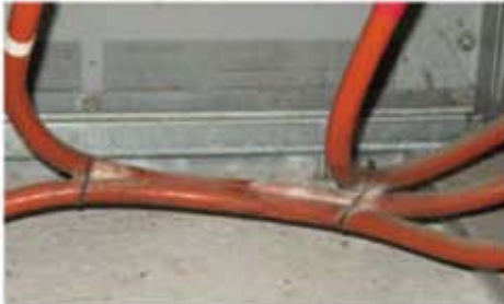
Figure 4 - White powder/dust residue formed on 13kV power cables that are tie-wrapped together forming tight air spaces between each other; ideal locations for corona to form.
