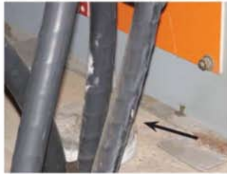
Figure 5 - 13kV power feed cables showing corona powder and a small but intense area of tracking (shown at arrow).
