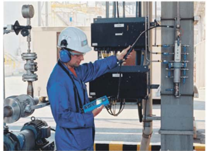
Figure 3 - Using a flexible sensor to find a compressed air leak on an instrument air line.
